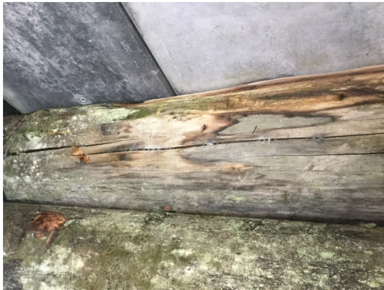
Horizontal crack on top face log right bank
