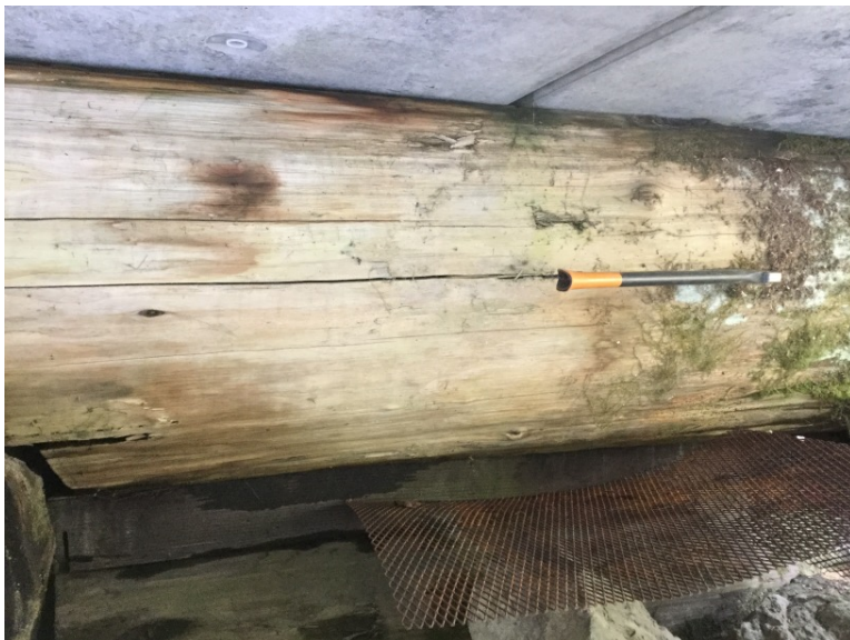
Horizontal crack on top face log left bank
