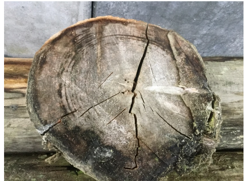
End splitting on tieback log at right bank
